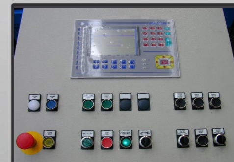
Painel de controle
