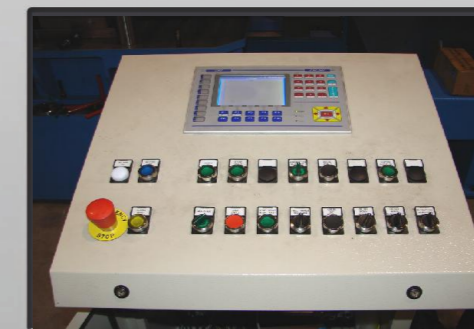
Painel de controle
