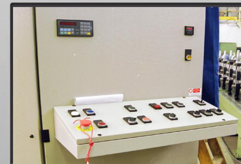
Painel de controle
